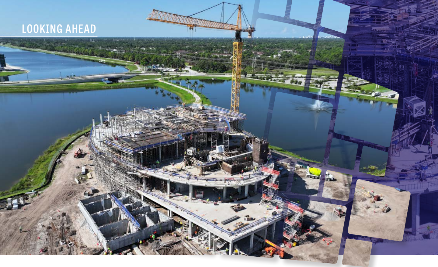
Above: An aerial view of the progress made on Mote SEA as of Sept. 15, 2023.
